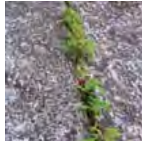
RESIST THE TEMPTATION TO REMOVE PLANT LIFE FROM CRACKS
